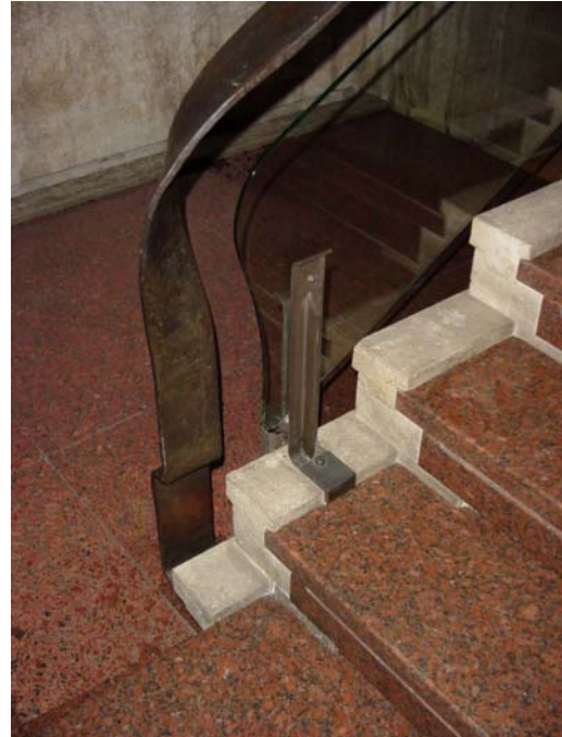
Figure 4: Detail of the Quaroni staircase, with the granite step embedded in travertine and the handcrafted handrail. Source: http://www.archidiap.com/opera/ristrutturazione-e-restauro-di-palazzo-orsini/ (Osmar).
